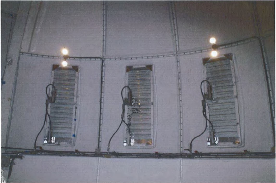
Figure 5.2 The inside of the dome showing three of the active vent gate assemblies. Visible on each of the vents are the two motors that adjust the damper settings.
